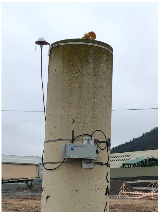
Figure 6: Installation of a base in a survey pillar. A prism for survey control has been installed on top of it and its position is being used as the base position for Loadsensing GNSS installation. The GNSS antenna has been installed within a certain distance from the radio antenna by using a 2,5 m cable
