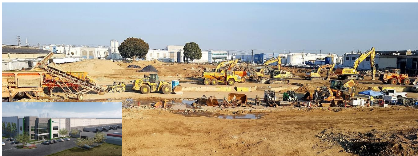
Building demolition complete, SCS Engineers performed soil remediation and associated dust monitoring services for the new industrial development in Los Angeles
